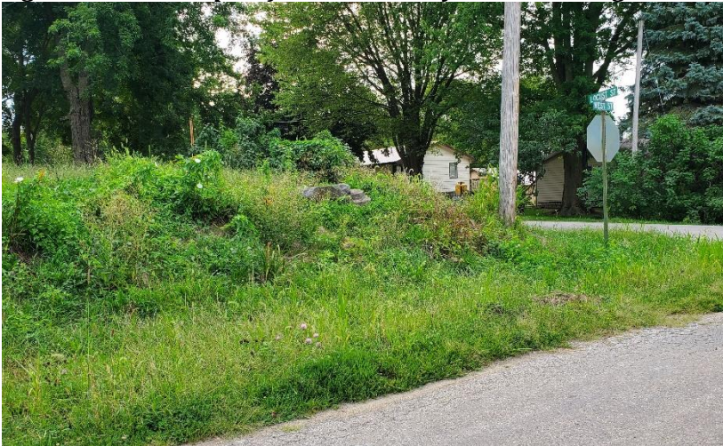
Figure 5-10: Example of Ditch that may become Overgrown
